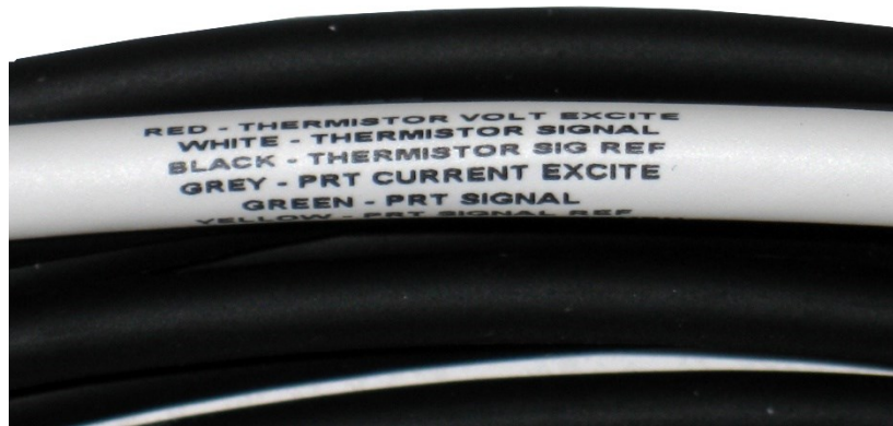
FIGURE 7-6. Labels on the pigtail end of the TEMP cable
